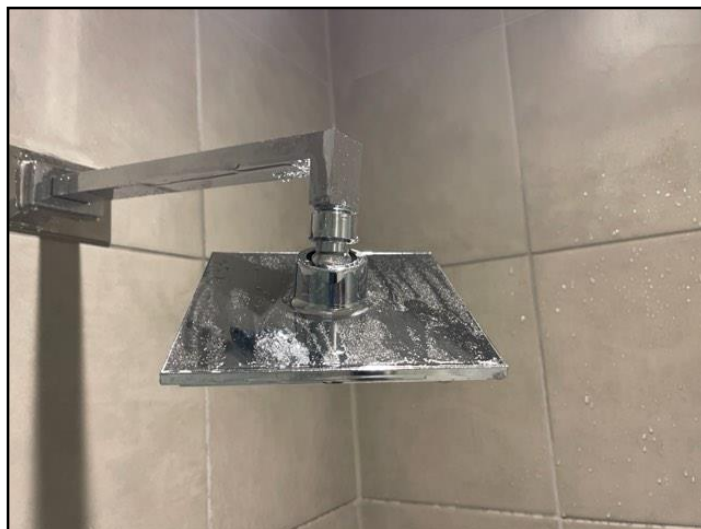
18. Shower head damaged
