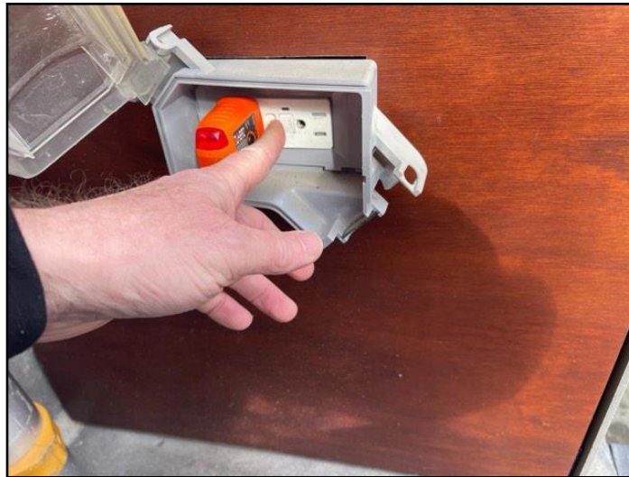
3. Test faulty on GFCI/GFI (Ground Fault...
