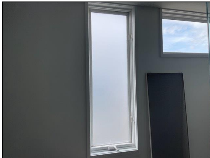
21. Difficult to operate
